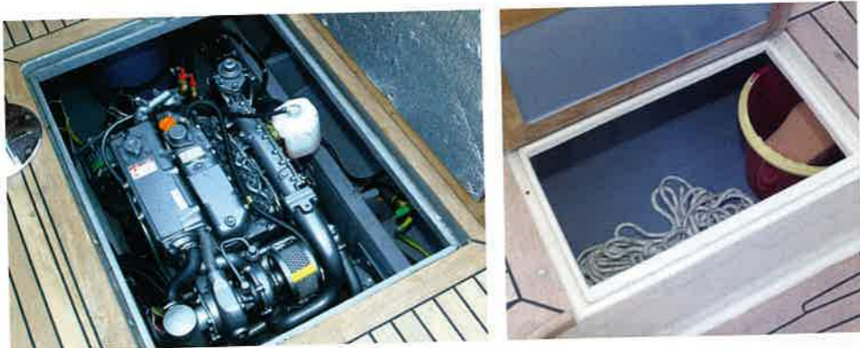
above The main engine hatch allows for servicing, but you can't climb in. Seat bases double as lockers.
