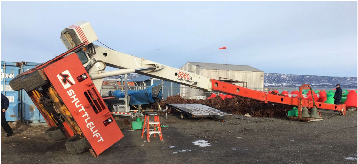
Overtured Mishap Crane
