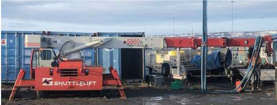
Mishap Crane after Righting with Outriggers Extended and Down
