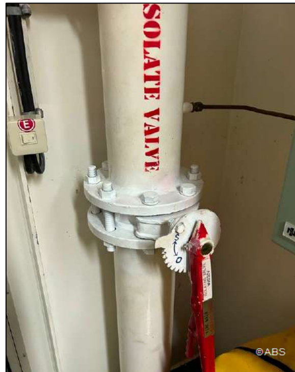
Main fire line isolation valve non-functional
