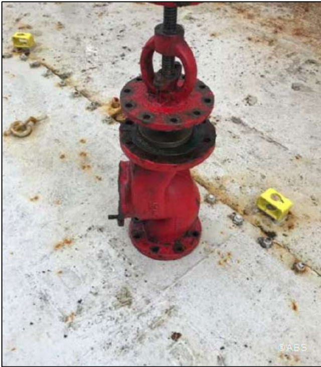
Engine room fire main isolating valve –malfunctioned
