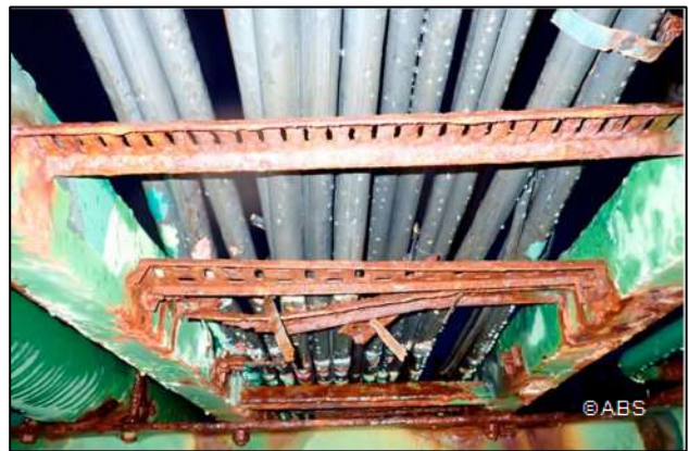
Corroded cable tray support on deck
