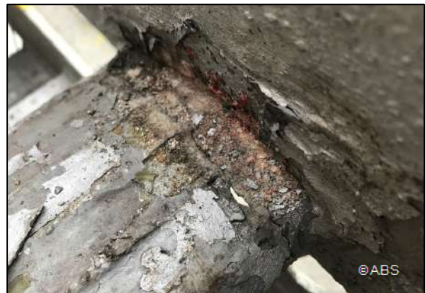
Crack accommodation ladder with waste
