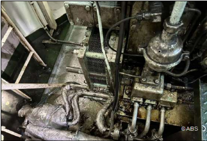
Generator engine fuel pipes leaking
