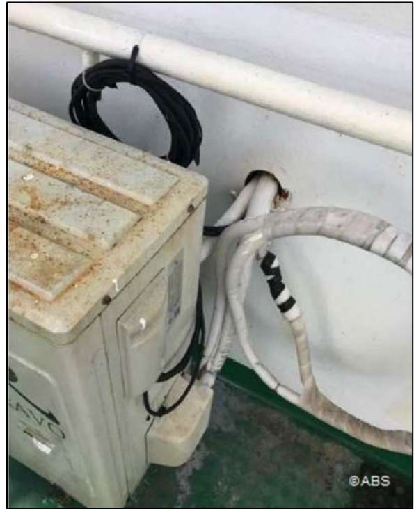
Bridge wing AC electrical cable penetration not approved type
