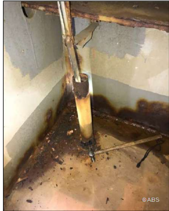
Wasted and broken electrical deck penetration with compound missing
