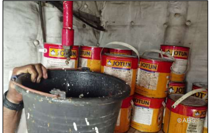
Paint store sprinkler head found clogged
