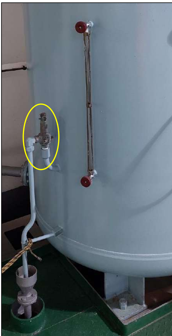
Figure 8: Safety valve to bilges
