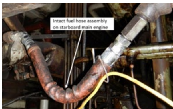
Flexible fuel hose assembly on the inboard side of the starboard main engine (Photo credit: TSB)
