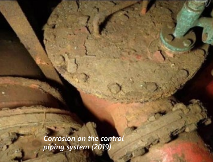
Deck of the FSO Safer, indicating the lack of basic maintenance (2019)
