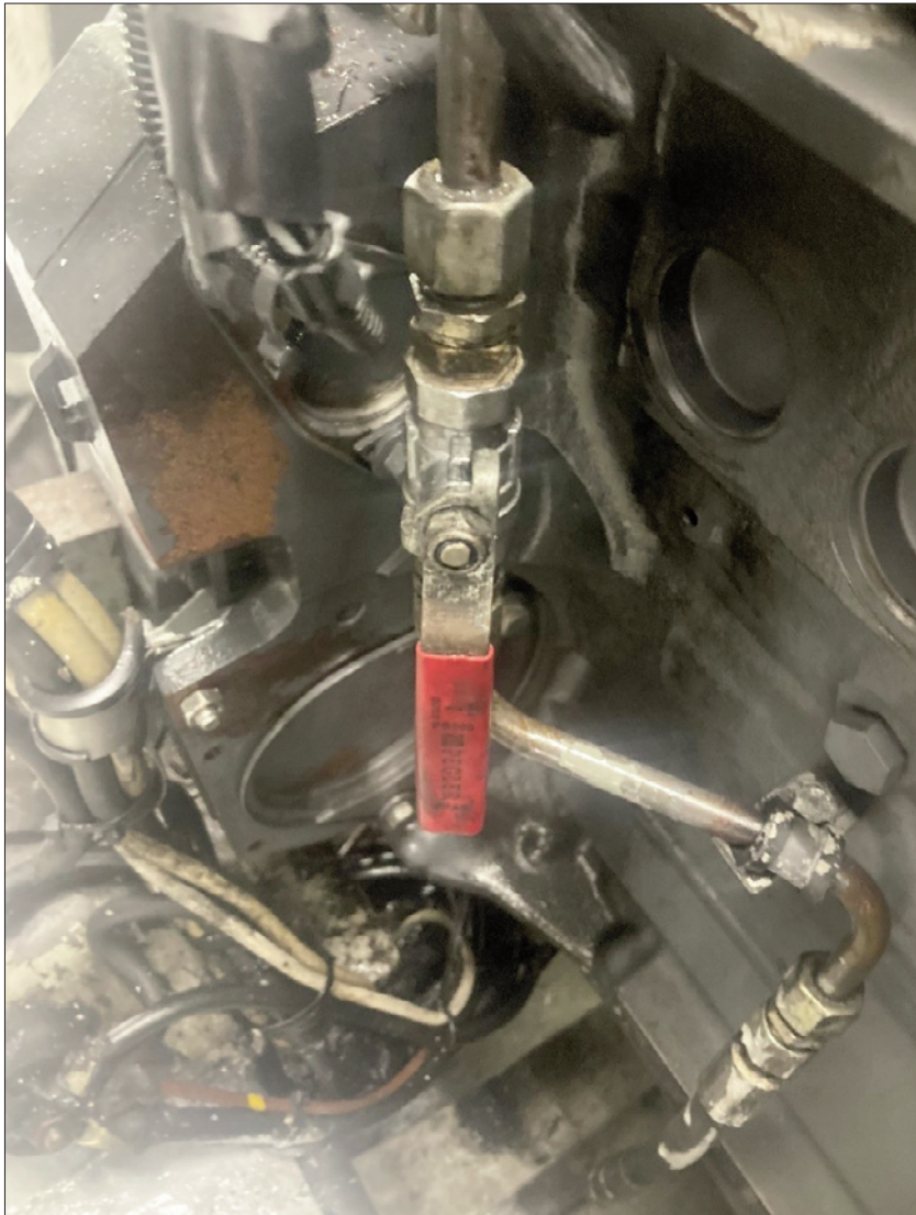
Appendix 7.3 Photograph No. 1 - Return Fuel Line Shut Off Valve
