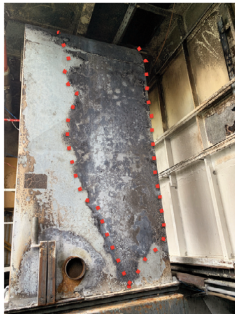
The Spray Pattern of Fuel & Flame Impingement on Air Intake Ducting
