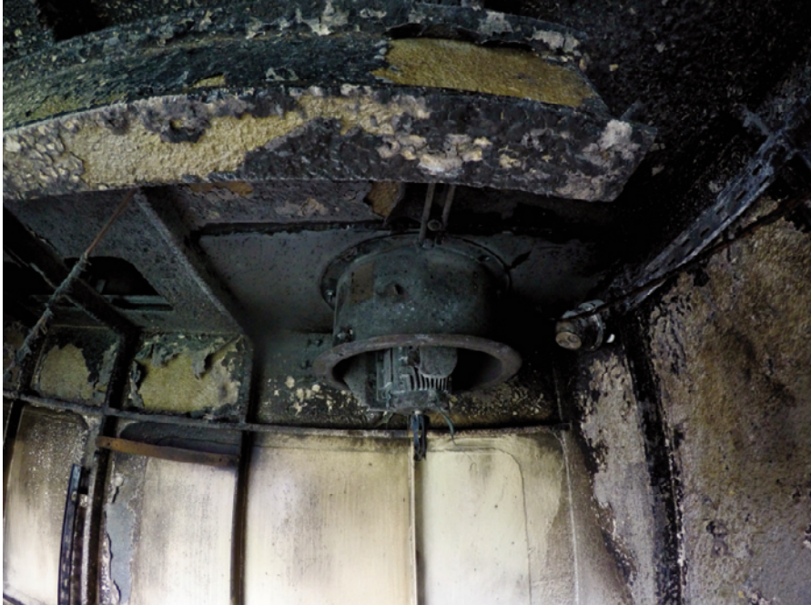
Photograph No. 10 – Flame Impingement on Air Ducting
