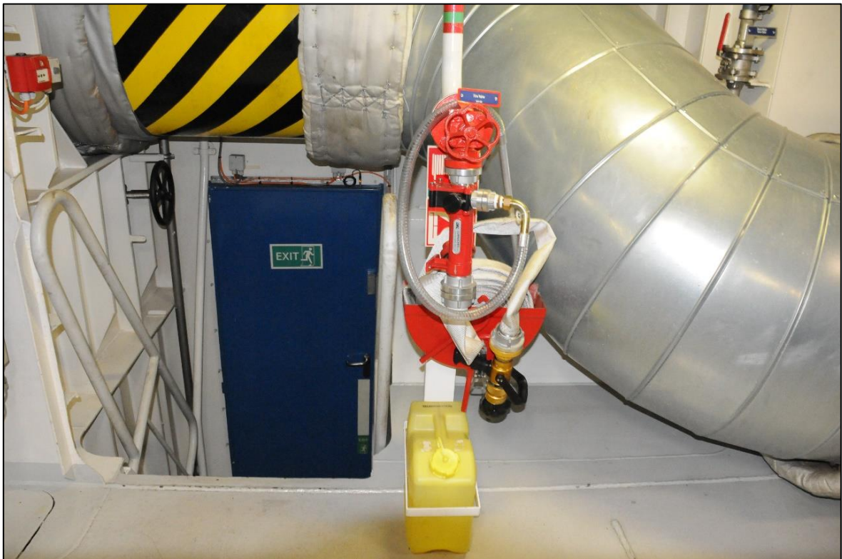
Figure 46: Hydrant station with foam/wetting agent
