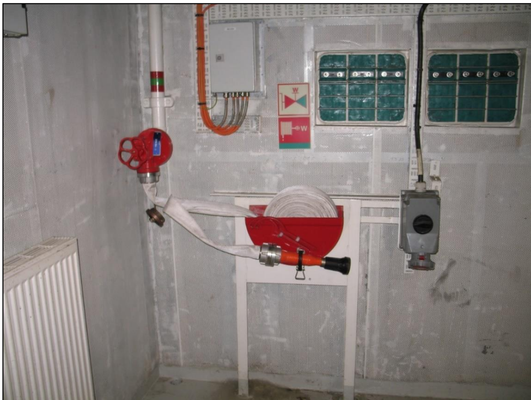
Figure 35: Equipment prior to fire
