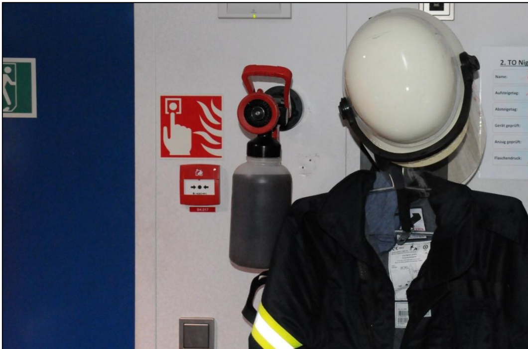
Figure 34: Venturi turbo jet pipe with 2 ltrs. of F-500 EA, for flexible initial attack in all engine-room areas, positioned in the Engine Fire Locker (firefighting equipment room)
