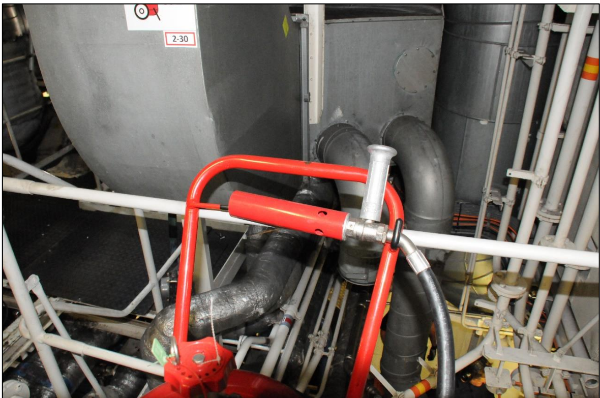
Figure 33: Low-expansion foam pipe (trolley) for incipient firefighting
