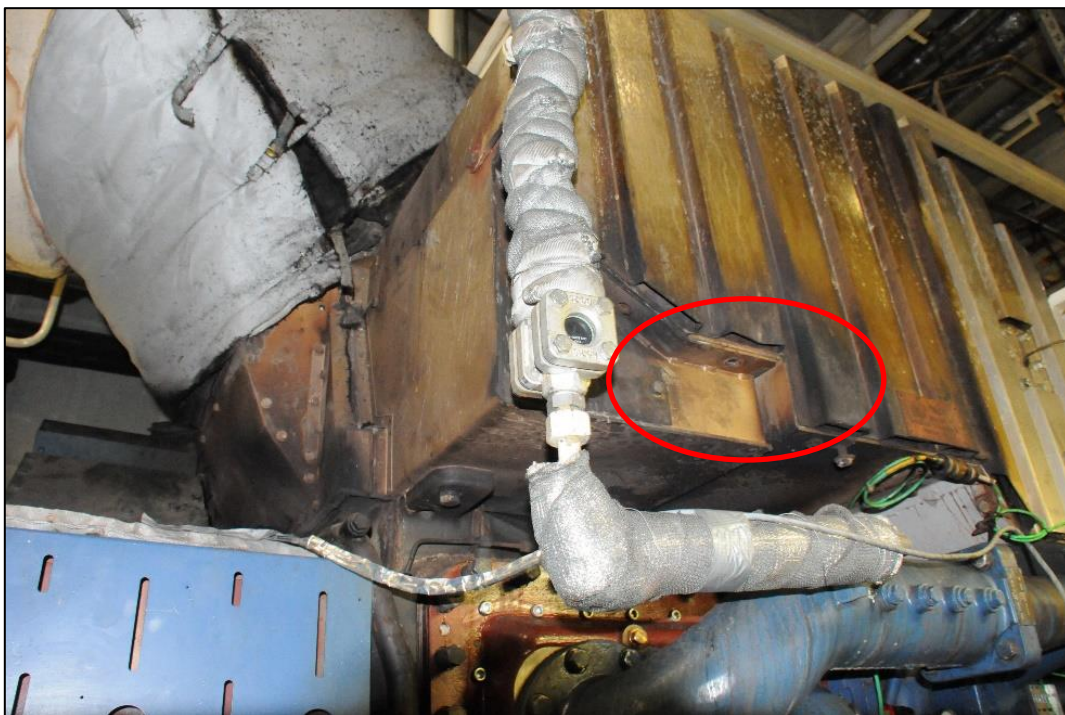
Figure 24: Burn marks on outside of turbocharger (exhaust side)
