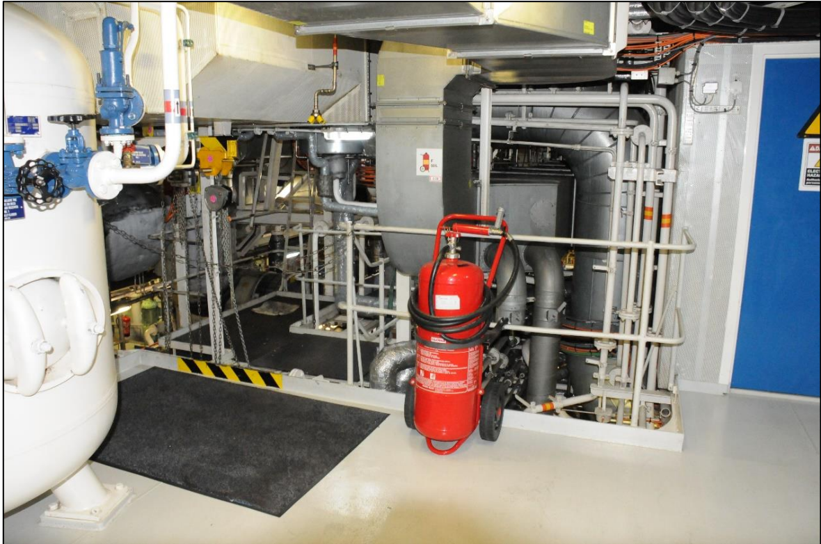
Figure 32: Foam trolley (in risk area)
