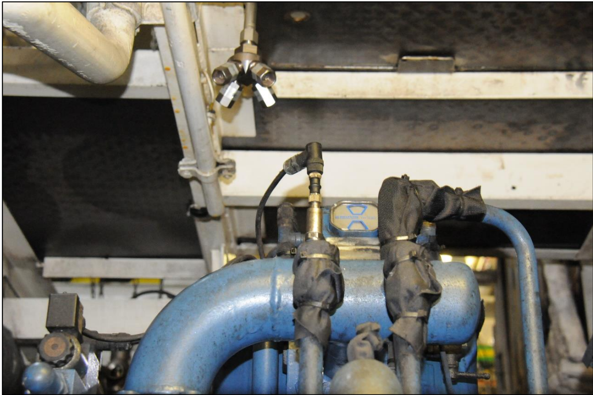
Figure 47: Pressure sensor replaced pressure gauge on top of gearbox
