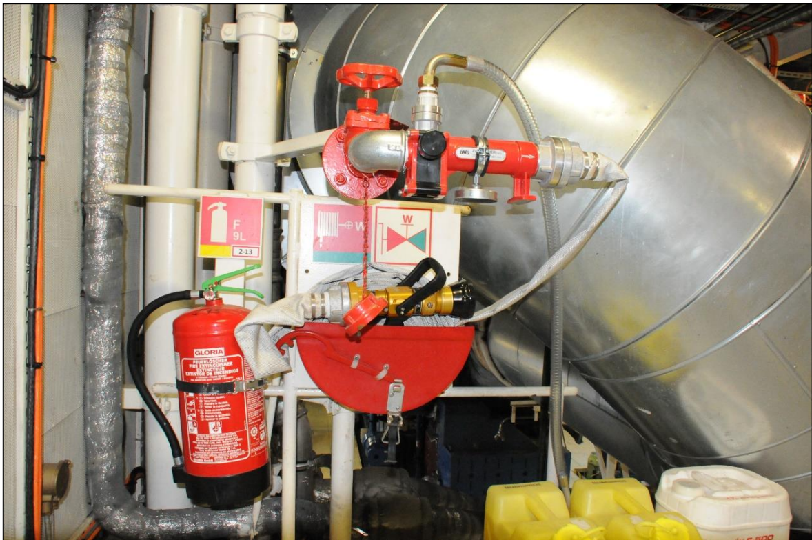
Figure 44: Hydrant station (risk area) with permanently installed admixture/inductor and turbo jet pipe
