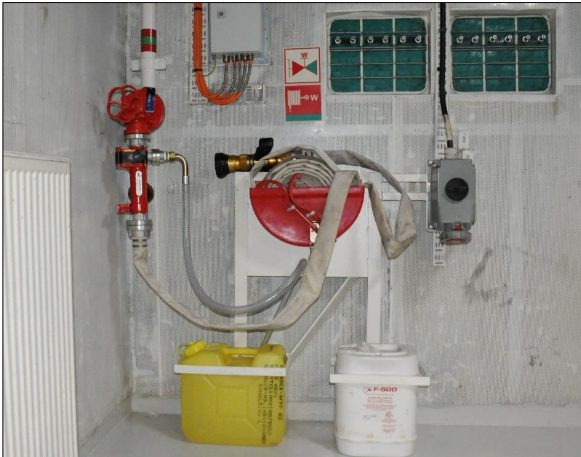
Figure 36: Equipment after fire
