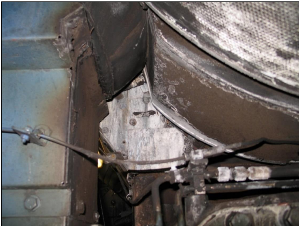
Figure 20: Fire damage to turbocharger insulation (air side)
