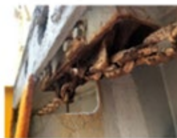
Corroded pulling chains for hatch covers
