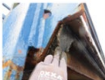
Deteriorated rubber packing near the edges
