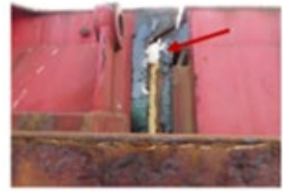
Foam between hatch covers
