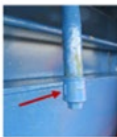
Drain pipe blocked
