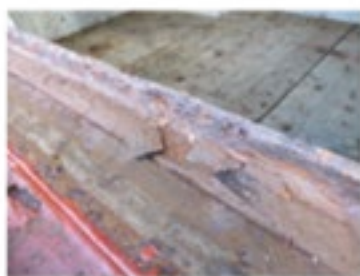
Corroded / wasted & uneven compression bar
