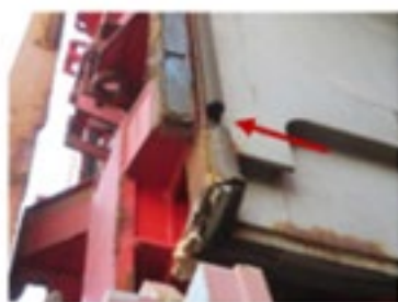
Gaps between insert repairs
