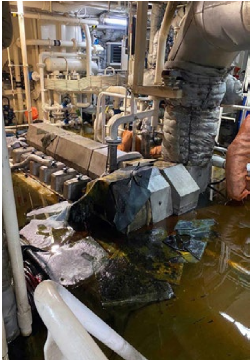
Figure 2: The flooded engine room
