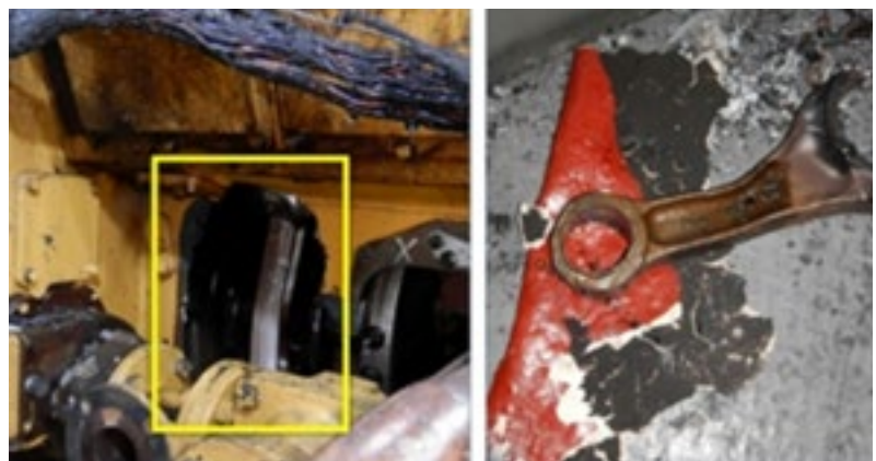
Damaged section of the engine (left) from where the connecting rod from the no. 3 DG (right) was ejected. (Credit: Oceaneering International).
