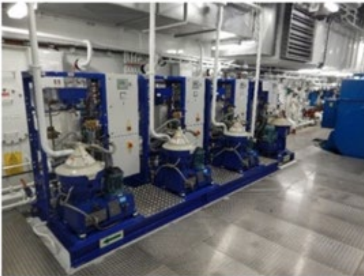
LO separator – MDO purifier rack
