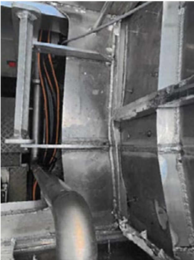
Figure 2: Deformed internal frames
