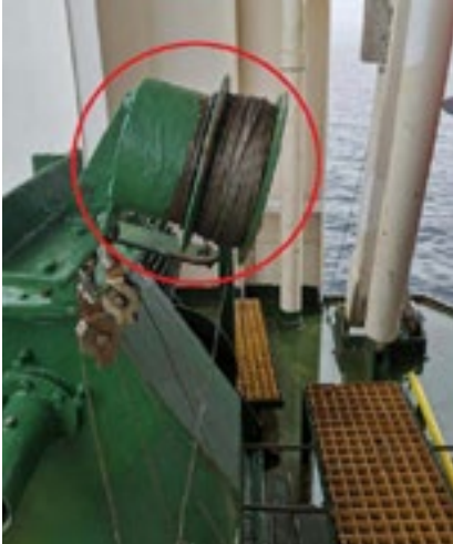
Brake release wire drum overpainted
