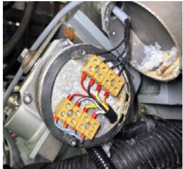
Figure 3: Water ingress damage (unrelated to the propulsion control loss)
