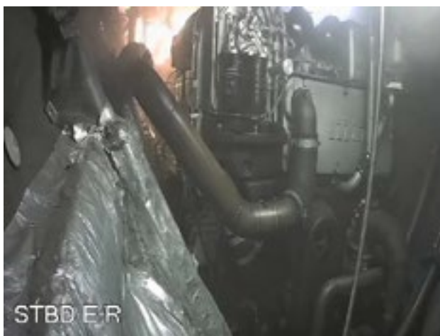
Figure 1: Engine fire seen on the CCTV
