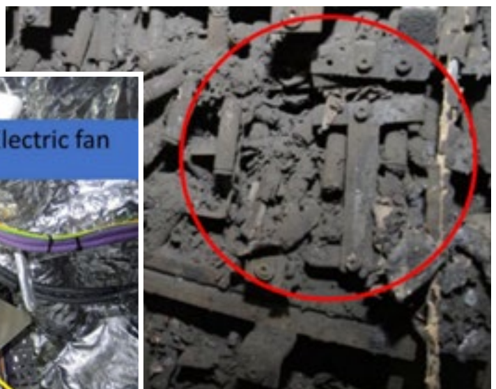
Remnants of battery module 2 in battery stack 6, with the copper strip encircled in red. Photo: Kripos
