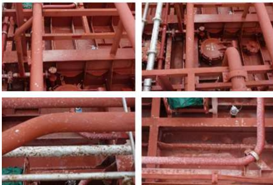
Figure 6 - Affected deck area
