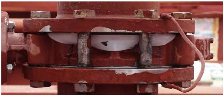
Figure 8 - Detail of damaged gasket
