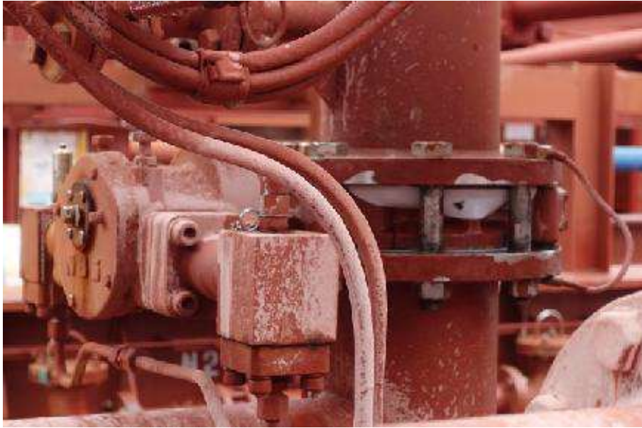
Figure 7 - Master valve of cargo only tank N°1P
