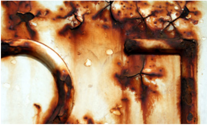
Corrosion is a concern for tank container owners and operators
