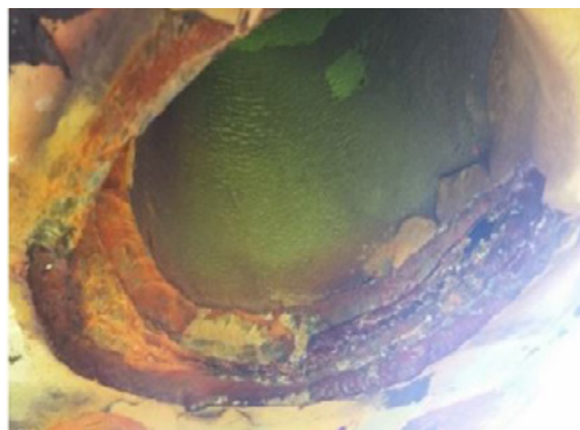
Cracks near distance piece leading to water ingress
