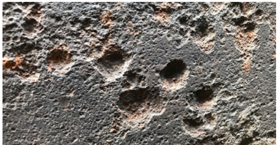
Photograph 3 - Contrast - Galvanic Pitting
