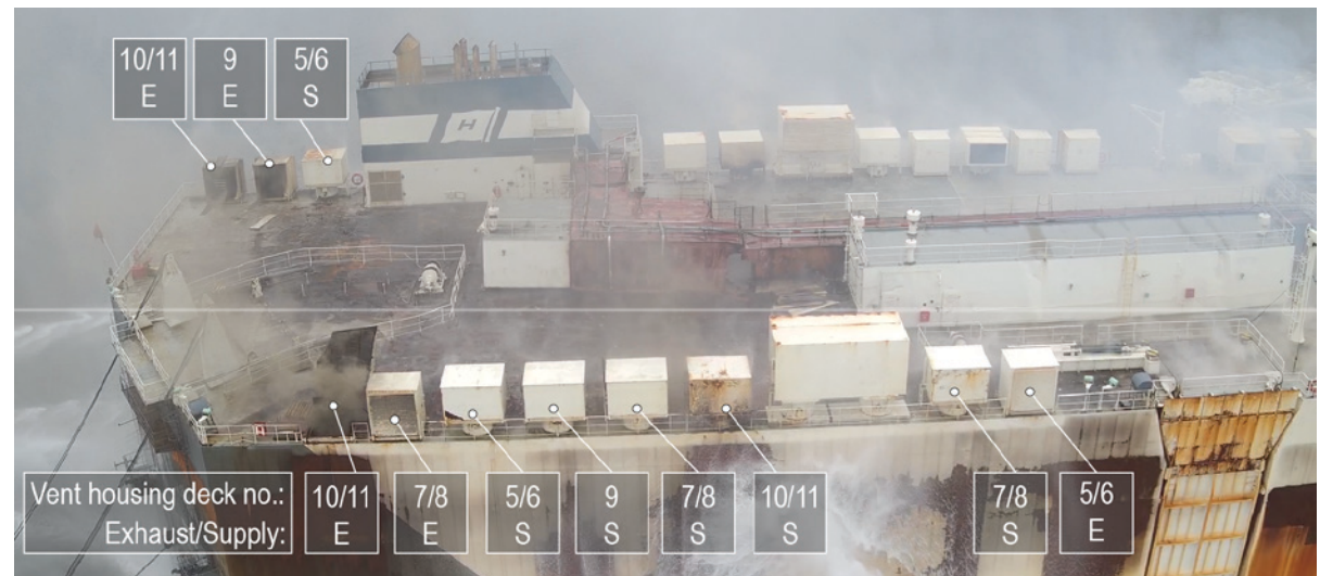
Figure 99. Damaged aft ventilation housings after the reported explosion of portside vent housing for deck 9 (9E in the photo). BACKGROUND SOURCE: JACKSONVILLE FIRE AND RESCUE DEPARTMENT
