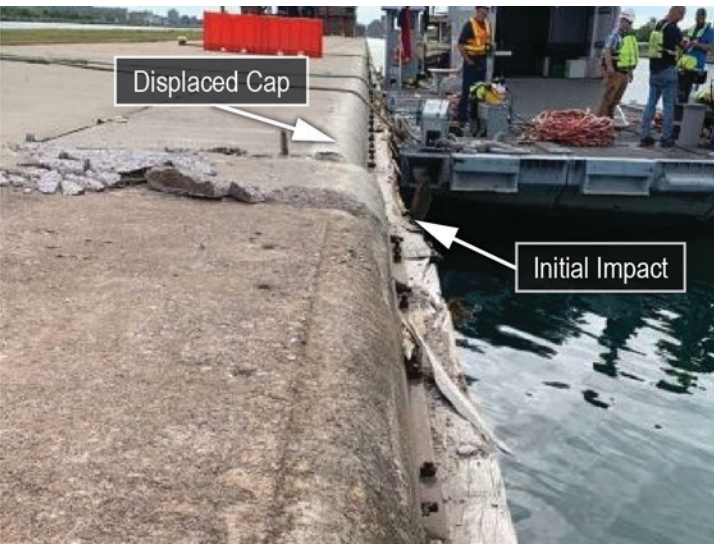
Figure 50. Postaccident photo of the west center pier. The location of initial impact is labeled and evident by a crushed timber fender. Displacement of a timber crib wall concrete cap is also labeled.
