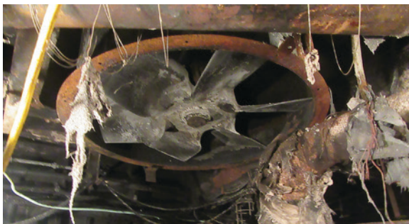
Figure 105. Starboard exhaust trunk fan (post-fire) located above the No. 1 generator. SOURCE: COAST GUARD
