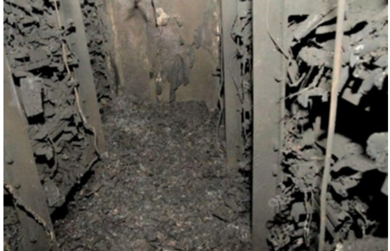
Fire damage to starboard battery room. Photo credit: Kripas
