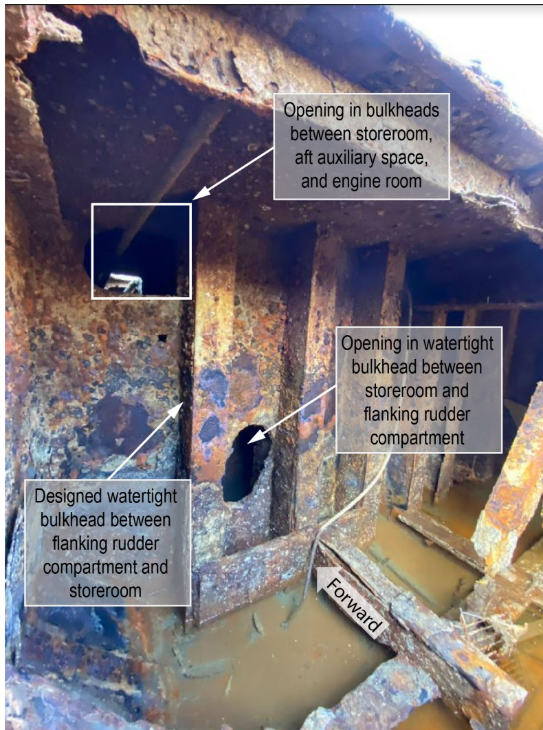
Figure 8. Flanking rudder compartment after recovery. Openings in bulkhead shown also typical of other bulkheads below the main deck separating compartments. (Source: Coast Guard)
