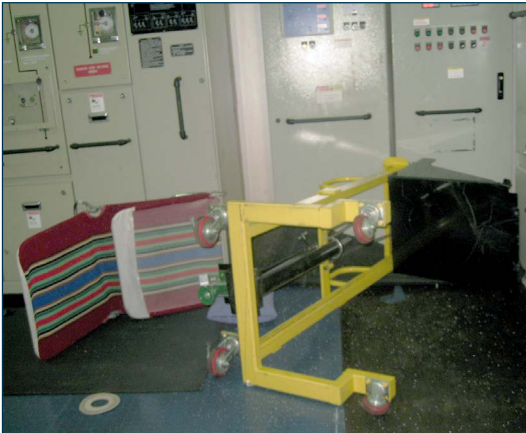
Figure 14: Overturned and displaced lifting device near control panels in the engine control room Source: Maersk A/S
