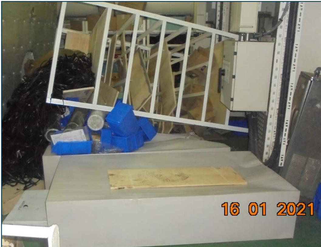
Figure 13: Overturned storage racks Source: Maersk A/S
