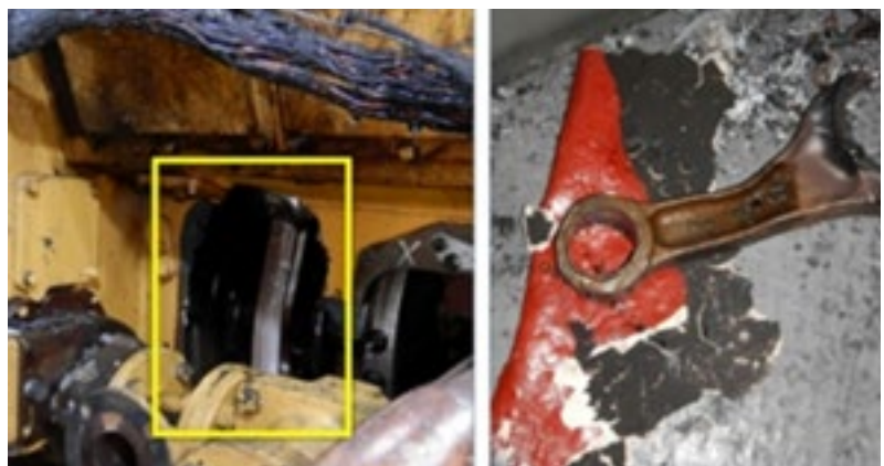
Damaged section of the engine (left) from where the connecting rod from the no. 3 DG (right) was ejected. (Credit: Oceaneering International).
