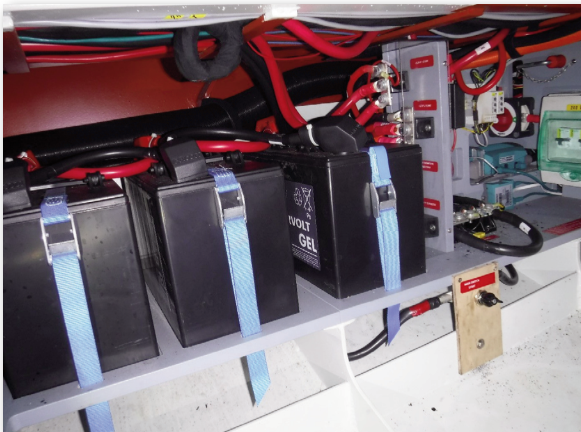
Appendix 7.4 After Starboard Corner of Engine Compartment (Image Taken of Sister Vessel)
