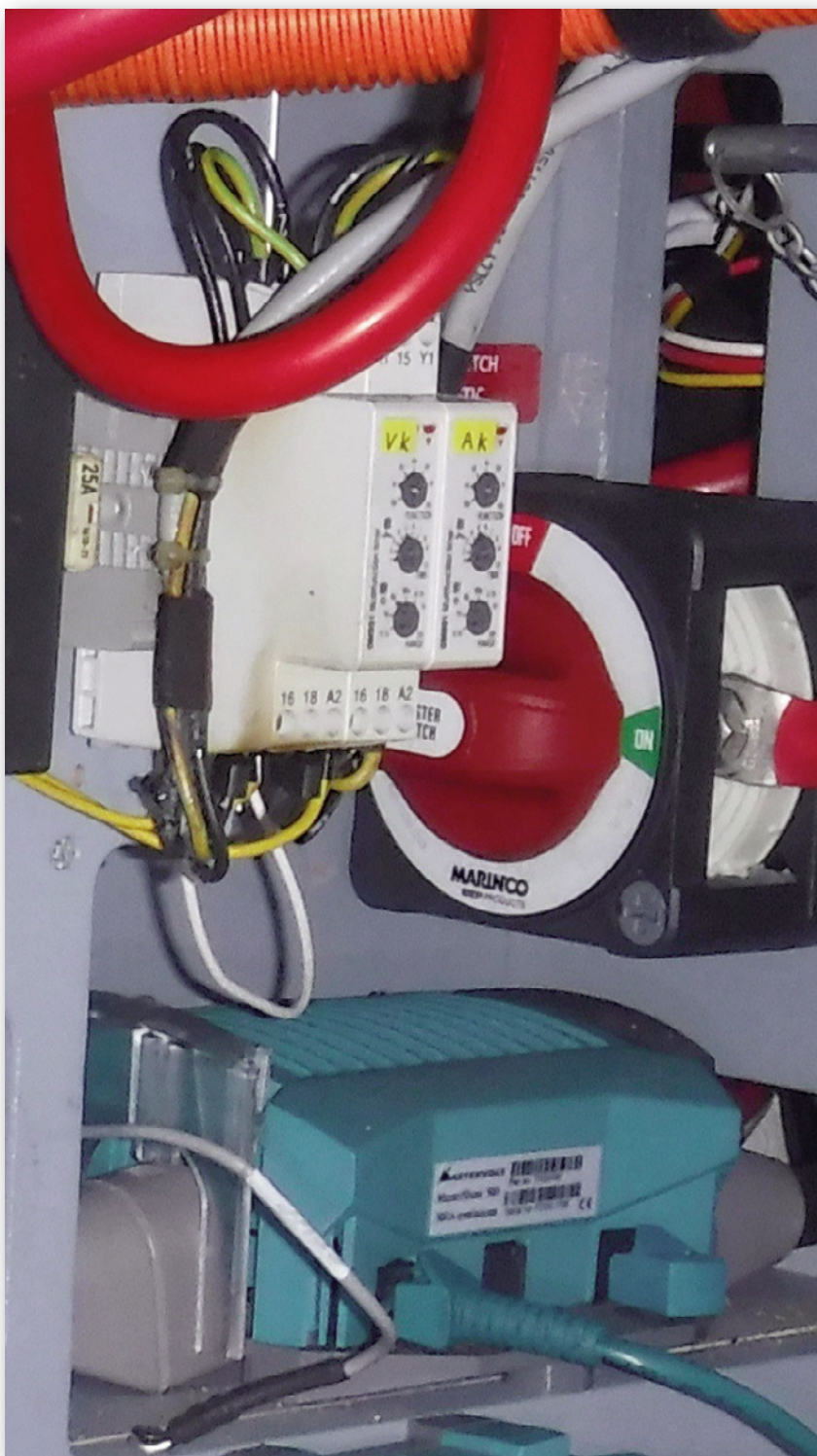
Appendix 7.12 Close Up of Isolating Switch and Timer Relay
