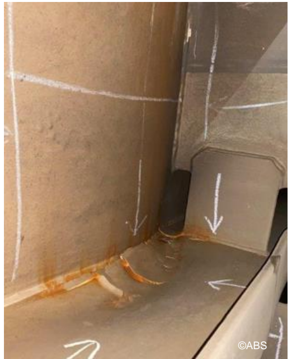
Internal structure buckled due to side shell contact damage
