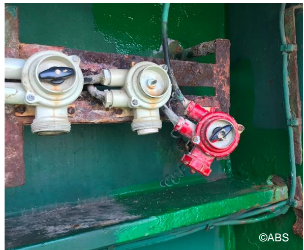
Damage to electrical installations
