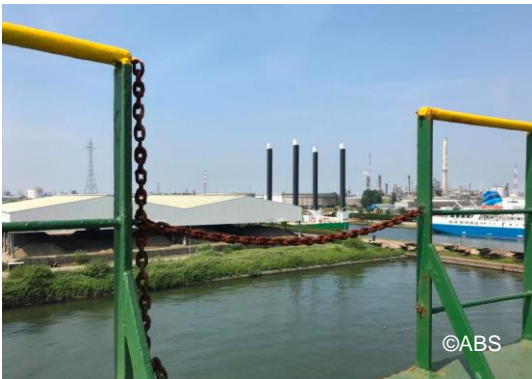
Missing chains for crew protection
