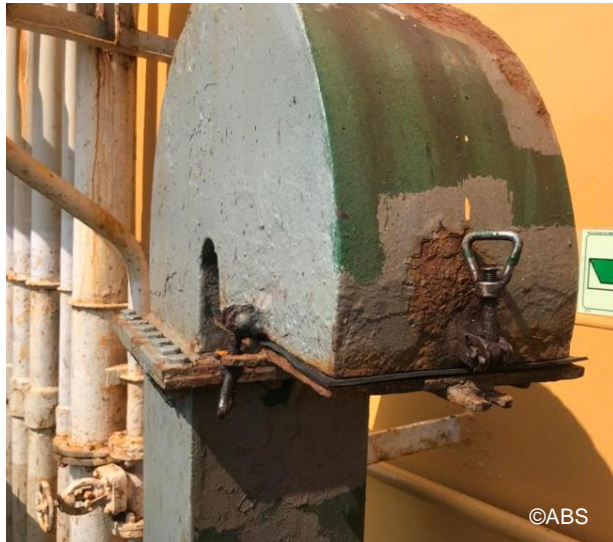
Ventilator found corroded - before
