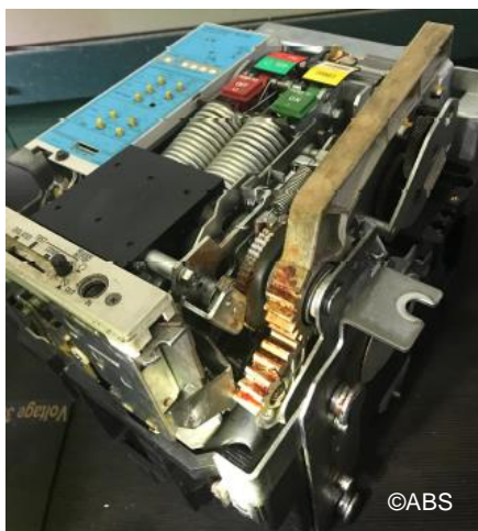
Emergency switchboard air circuit breaker damaged
