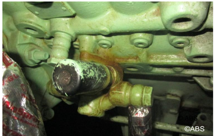
Emergency diesel generator high pressure pipe leak
