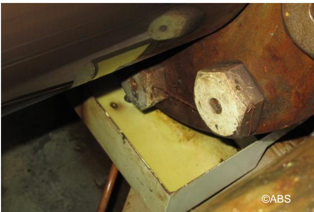
Steering gear leaking oil
