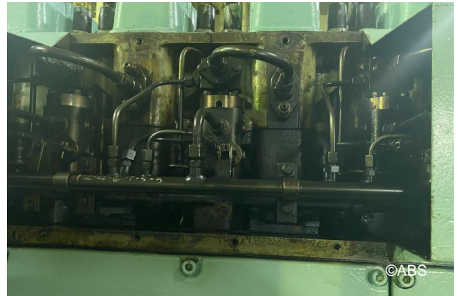
Main engine fuel pump leak
