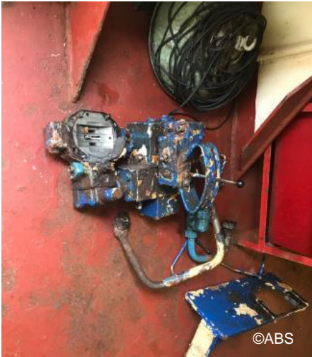
Damaged hydraulic motor for mooring winch removed
