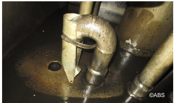
Funnel area – oil spillage from tank airpipe
