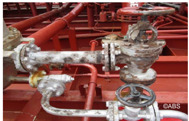
Steam pipe found with corrosion
