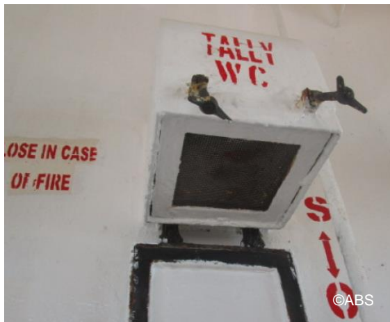
Ventilator dog broken/missing
