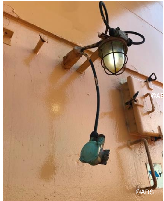
Damage to electrical installations
