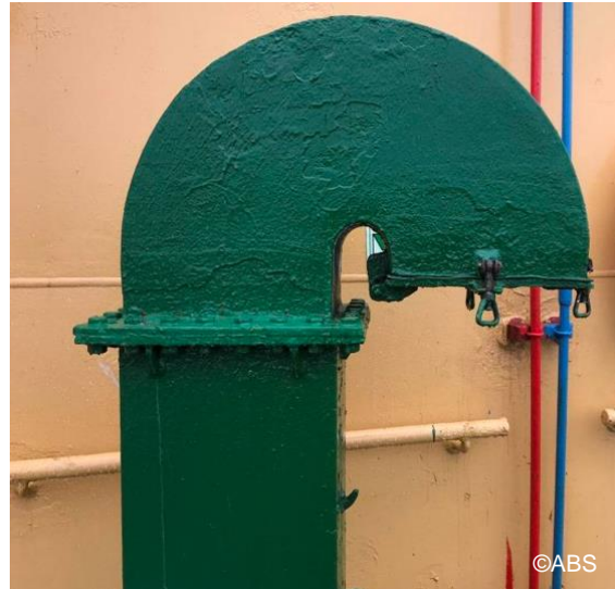
Ventilator found corroded – after
