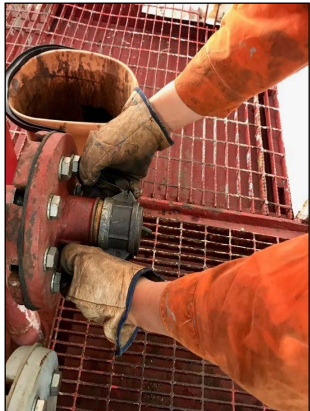
Figure 3: Reconstruction of the removal of the blanking plate when the system was pressurised
