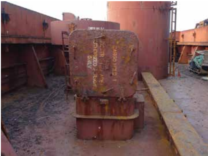
Figure 2.11 | Cargo hold access hatch in poor condition.
