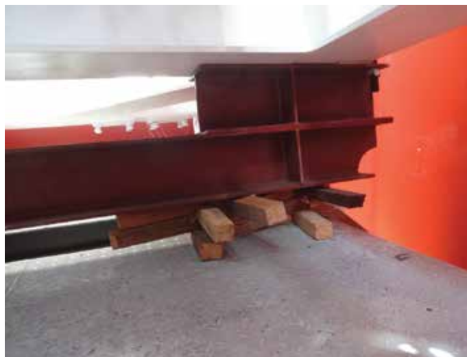
Figure 4.8 | Crushed dunnage due to improper arrangement.
