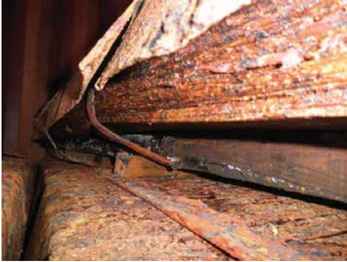
Figure 1.7 | Heavily rusted steel slabs.
