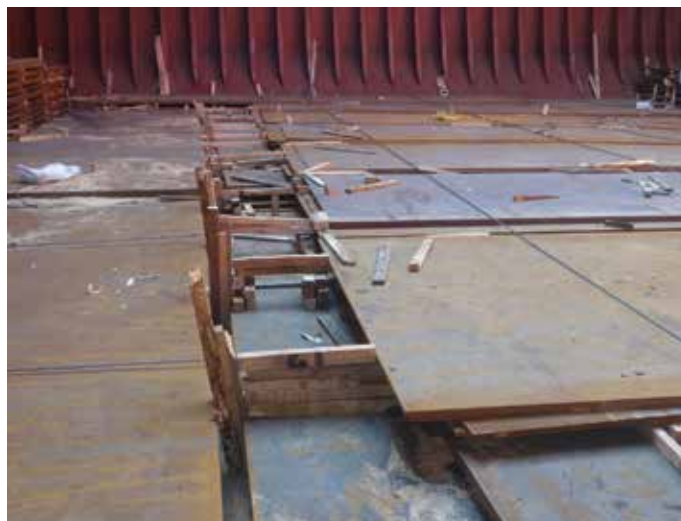
Figure 5.27 | Gaps between steel plates should be properly chocked before the vessel sails.
