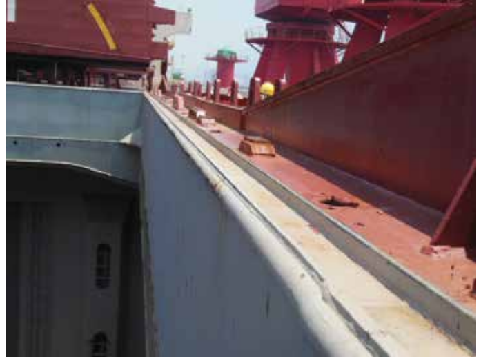
Figure 2.2 | Water drainage channel, compression bar and the landing pads as shown in good condition.
