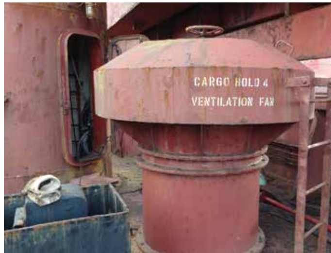
Figure 2.6 | Cargo hold mechanical ventilator.
