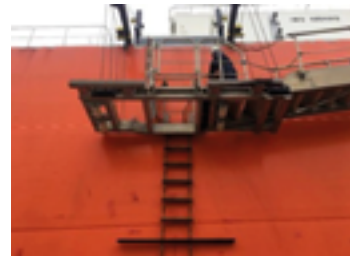
Non-compliant trapdoor arrangement.
