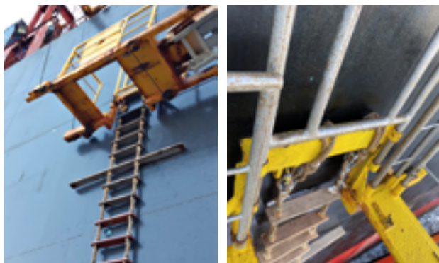
2 examples of non-compliant 'trapdoor' pilot boarding arrangements
