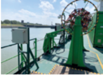
Non-compliant (by design) pilot ladder winch.
