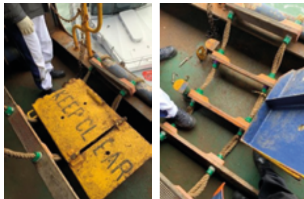
Looks like a safe access but the 3cm piece of steel is the only thing between life or death.
