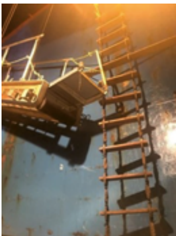
A non-compliant combination arrangement.
