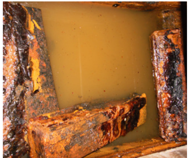
Fig 7. A rusty bilge seen on an older steel narrowboat. No other access was possible to check the condition of plating from inside the vessel. Needless to say the black steel was unpainted and badly pitted inside and out.
