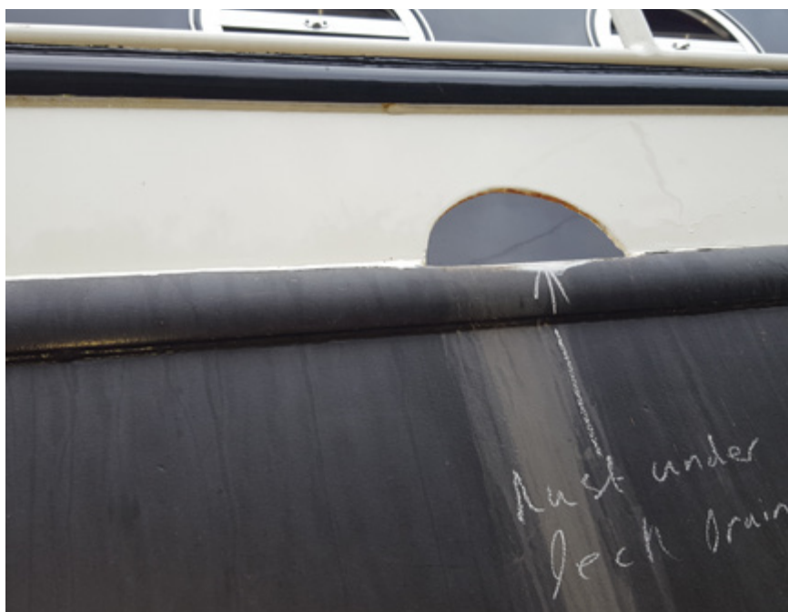
Fig 10. The one water freeing port in the solid bulwark which was also showing symptoms of corrosion.
