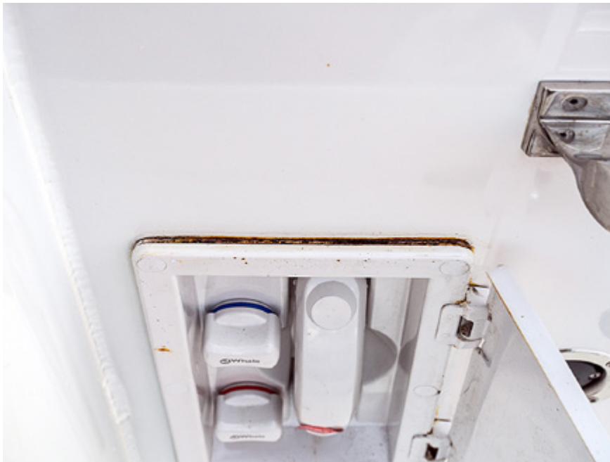
Fig 14. Rust around an external shower fitting owing to unprimed cut steel edges.
