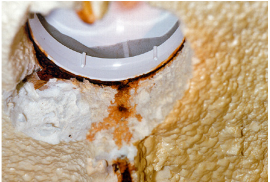
Fig 11. Unprotected steelwork corroding around a deckhead ventilator behind spray foam.
