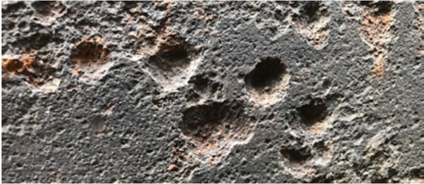
Photograph 3 – Contrast – Galvanic Pitting
