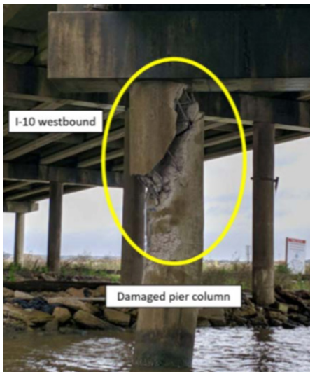
Figure 3 | Damaged bridge column
