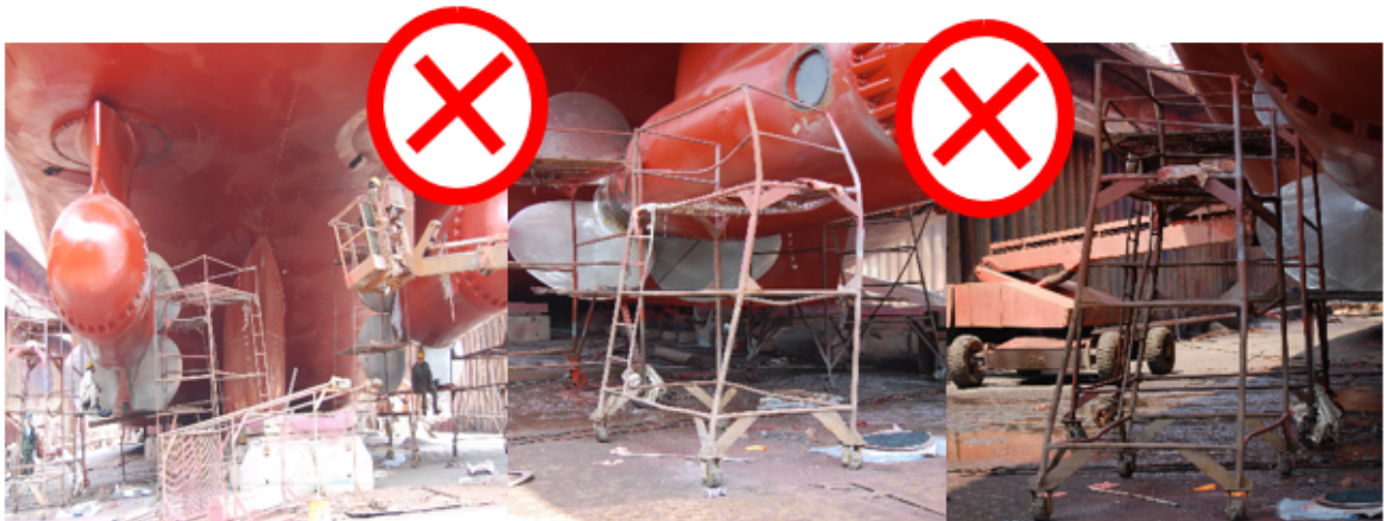
Figure 16.2: Damaged and dangerous mobile scaffolding
