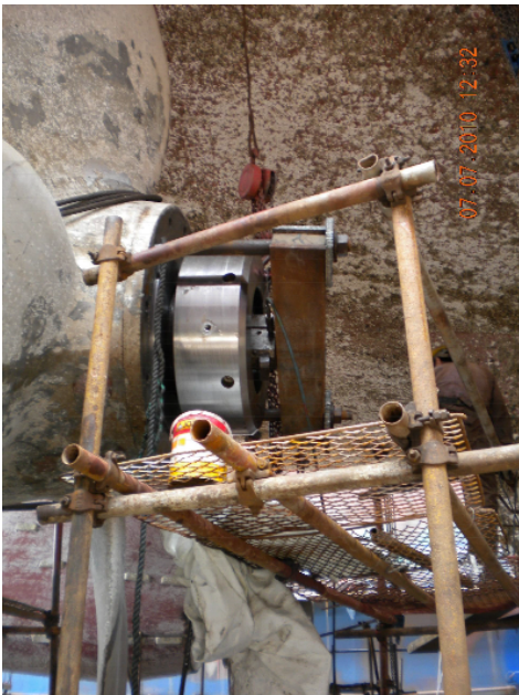
Fixed scaffolding in dangerous state
