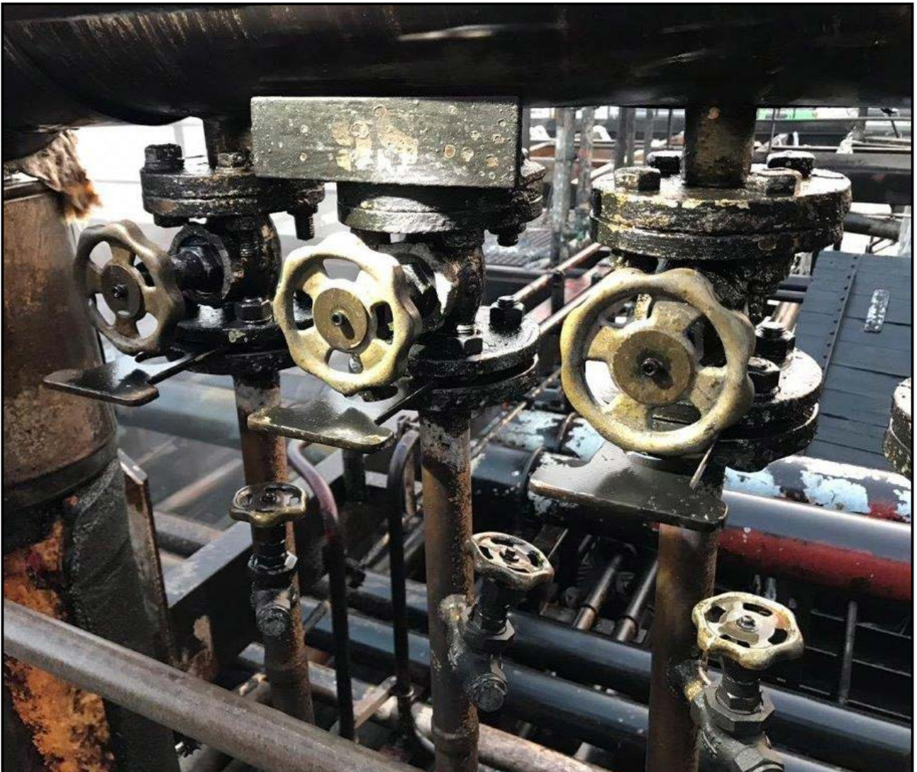
Figure 10: 9S heating control valves
