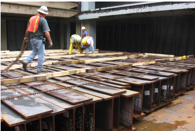
Figure 31: First tier of nested I-beams stowed in the hatch square. Tightly stowed I-beams are secured with chains to deck fittings
