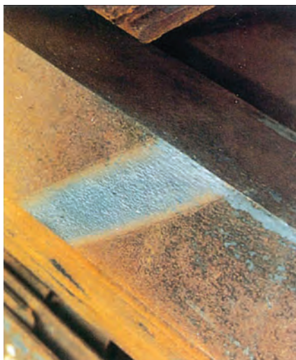
Fig. 1. Channels and angles (rust cleaned away locally). Surface-condition clause: rust stained
