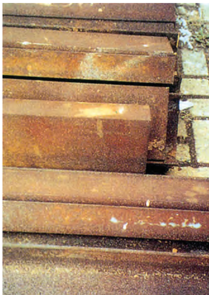
Fig. 9. Channels. Surface-condition clause: rusty
