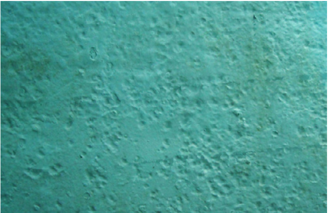
Photograph 1 - Galvanic Pitting on a (Painted) Mild Steel Hull in Fresh (River) Water
