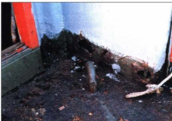
Photograph 1 Corroded accommodation house side structure
