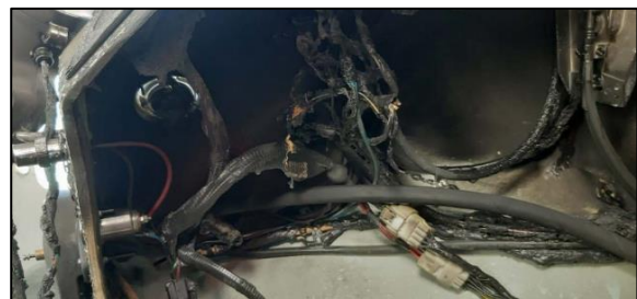
Figure 6: Damaged power cables under control panel
