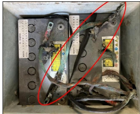
Figure 8: Cable in the suspecting short-circuit loop position
