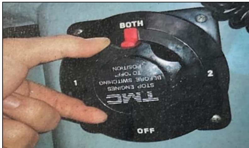
Figure 3: Battery changeover switch
